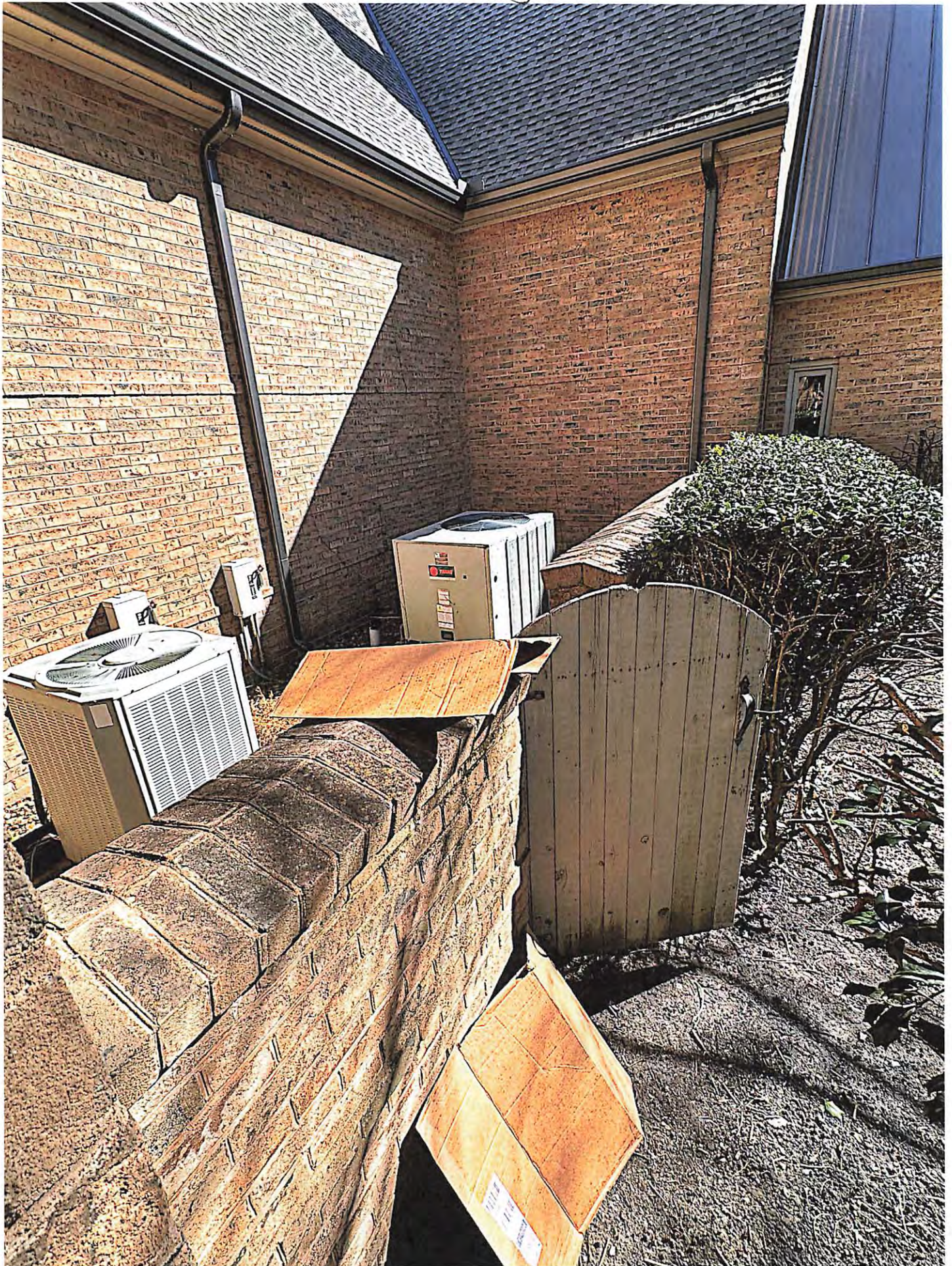
closer view of N. Academy St HVAC Corral
