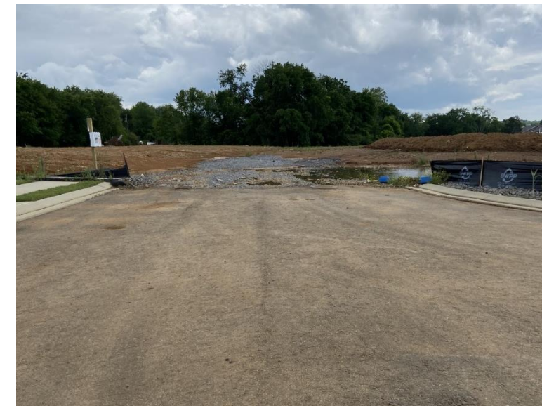
PHOTO 5: RIVER DOWNS ANNEX CONNECTION LOOKING SOUTH
