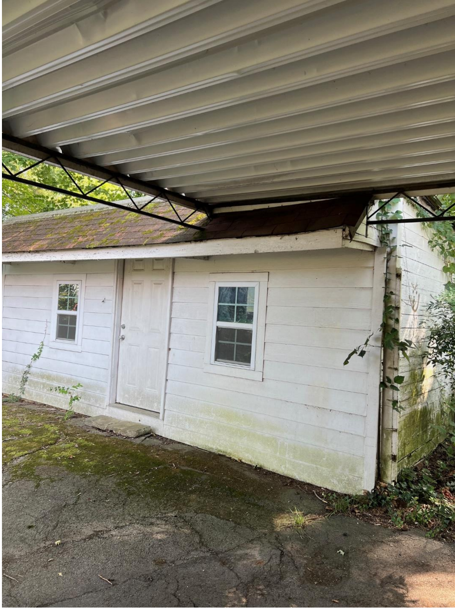
Closer view of storage building with attached carport. Building site will be re-graded to match current grade of driveway and yard.
