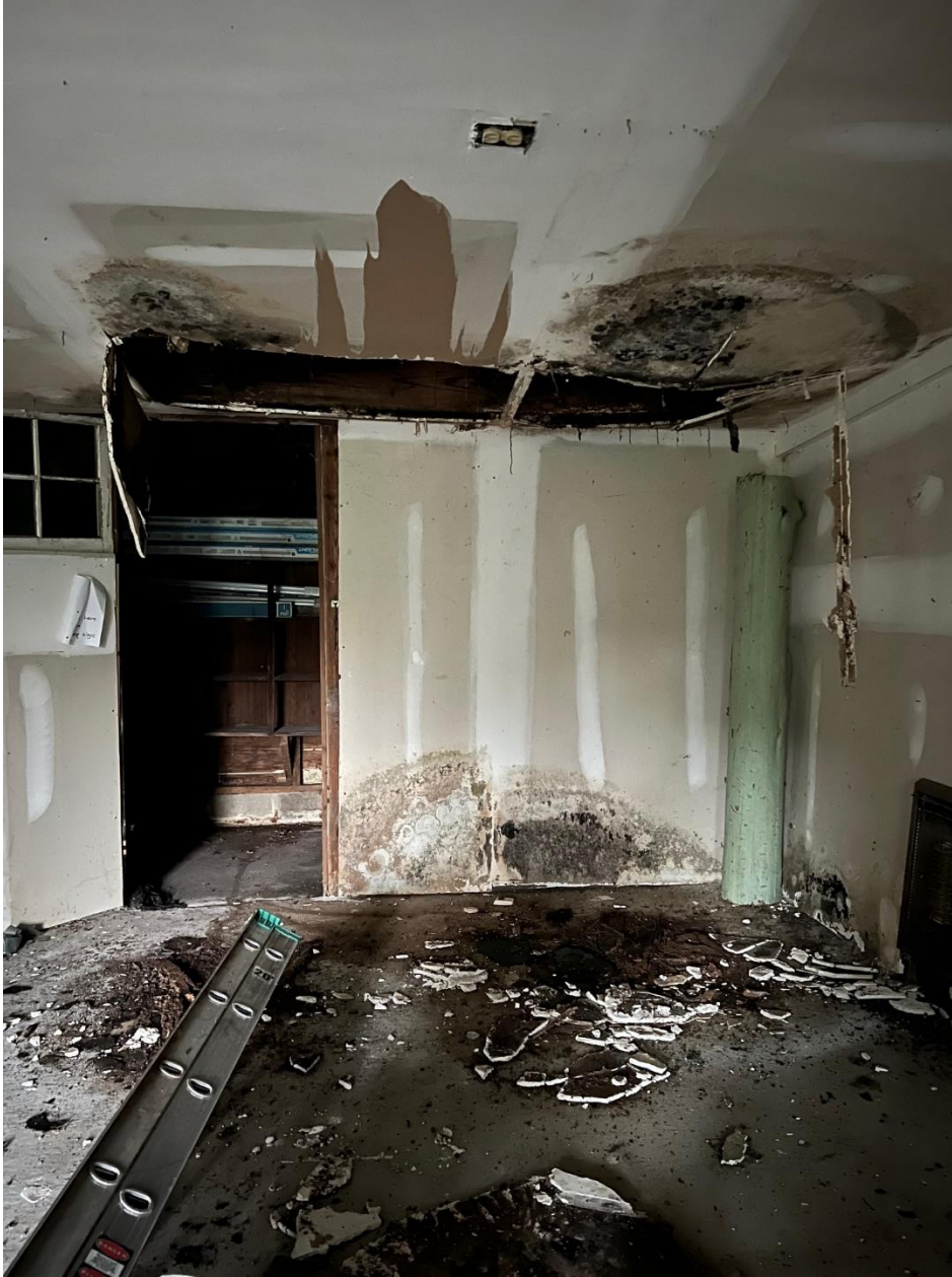
Inside view of storage building showing roof & ceiling collapse.
