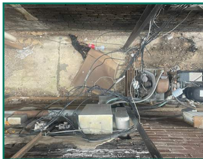
IMAGES OF EXISTING ELECTRICAL UTILITIES
